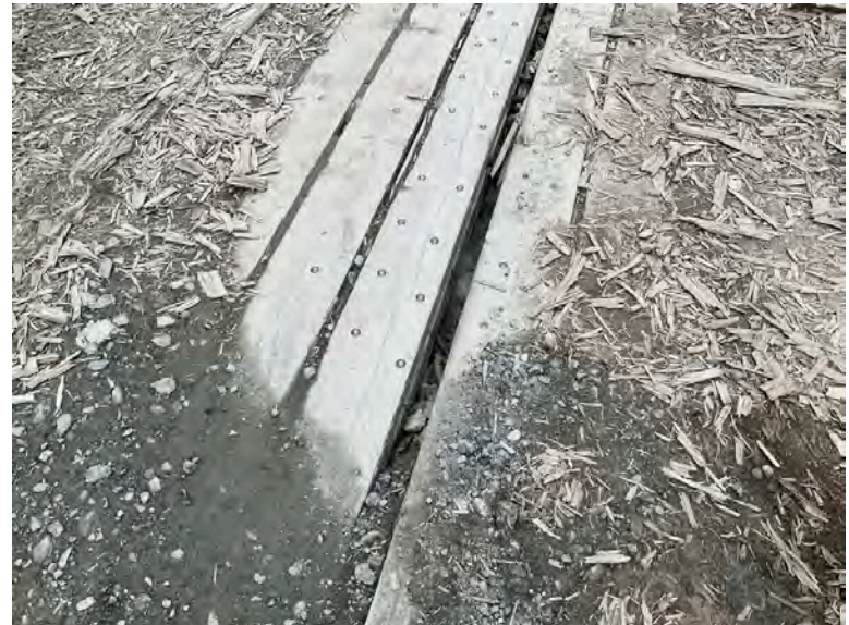
Gap under subdeck
