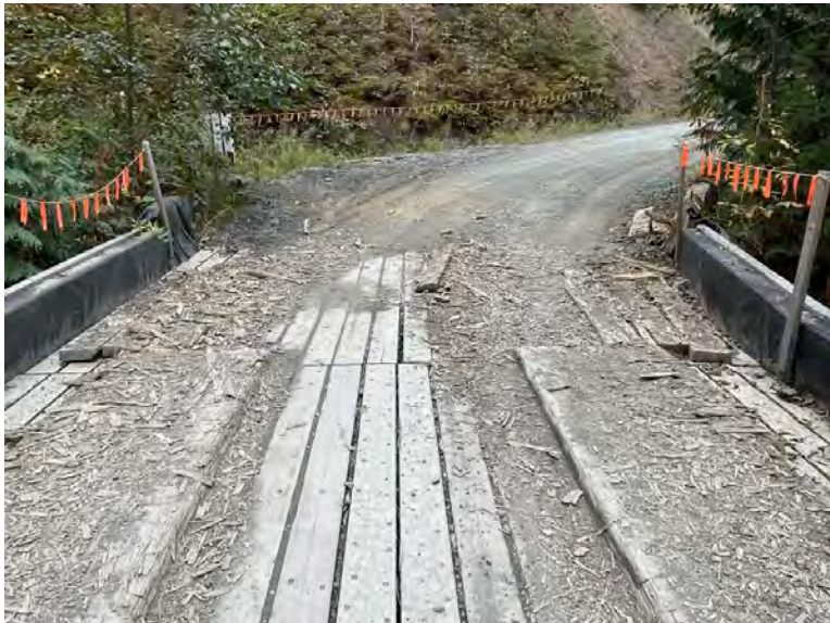
Running plank condition at ends in poor condition
