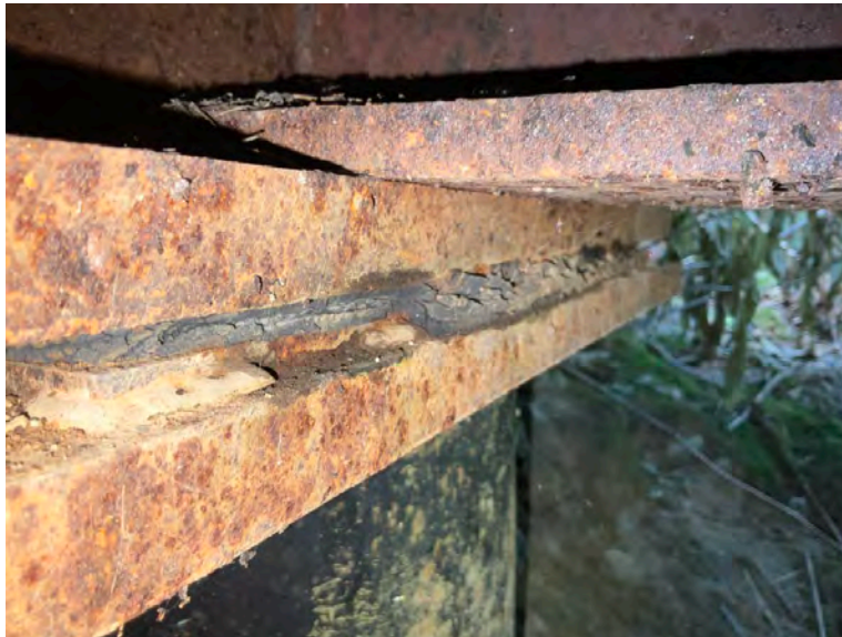
Rubber bearing pads deteriorating on stream side face, left bank
